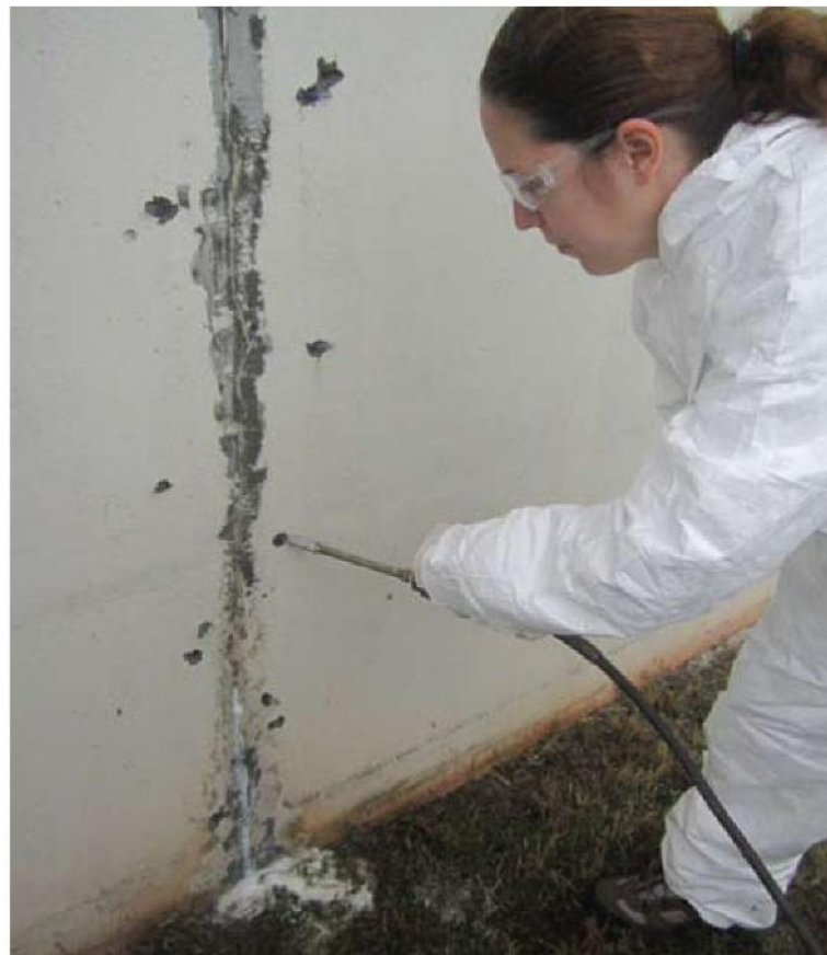
Christine Villano of Basement Solutions of the Hudson Valley injecting high pressure expanding polyurethane foam into cracks to seal off water from recent storm damage and flooding.
